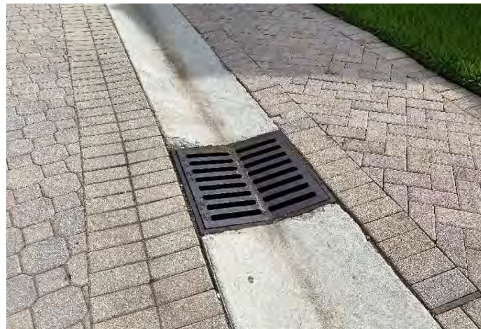
Storm Water Drain Catch Basins
