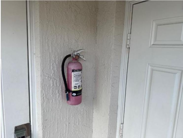
Photos / Fire Protections
